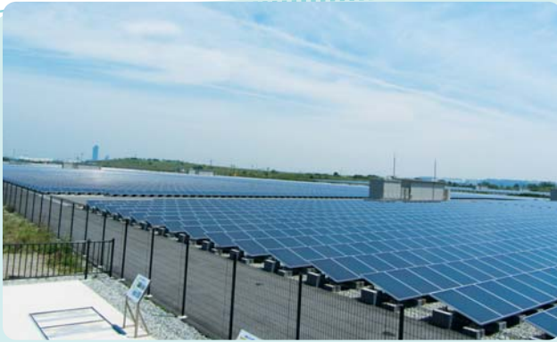
The large scale solar (photovoltaic) power station called "Mega-Solar" at Sakai city
